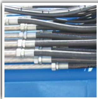
HYDRAULIC STAINLESS STEEL PIPING
